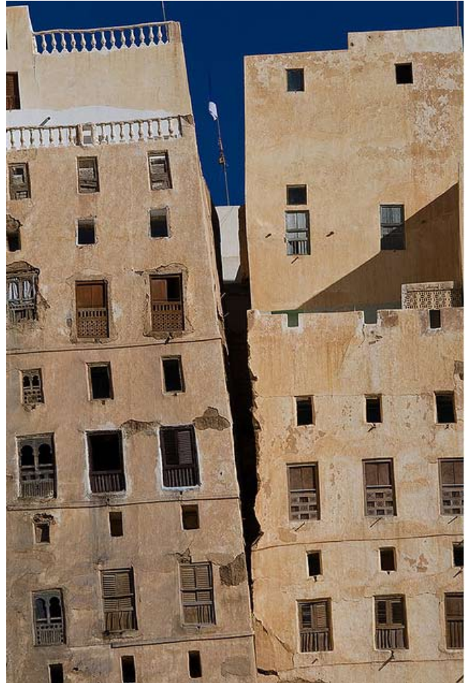
Fig. 12. The gap between the upper parts of two buildings in Shibam. https://secure.flickr.com/photos/phil_mari-on/4069822322/in/set-72157605482941019 .
